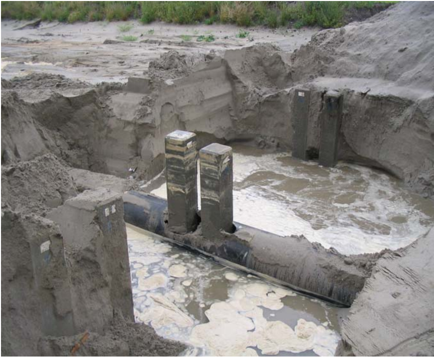
Photo 1: example of an incident: contractor has pinched the water pipeline
